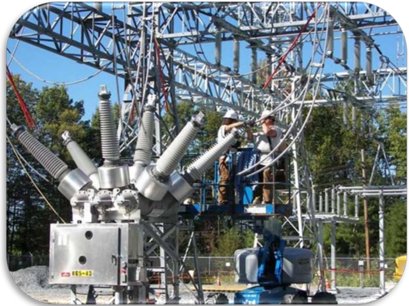
VELCO- Queen City 115 kV Substation Breaker
